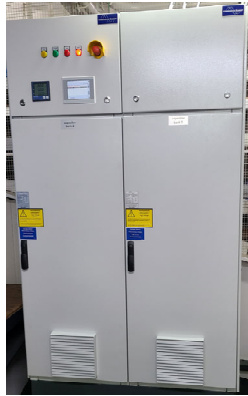
Fig. 3: RESI resonance elimination filter for 6,6 kV
